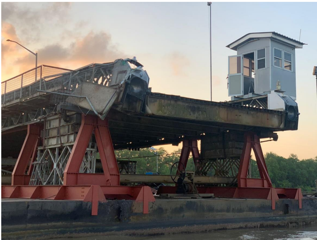
Image 3 - Damaged section of the retractor span
