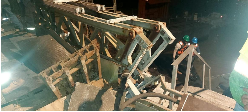
Image 2 - Damaged section of truss deck on Span 8
